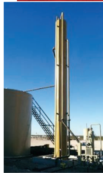
Vapor Recovery Tower
