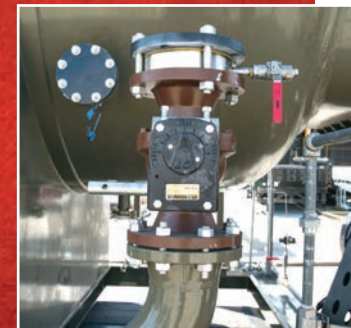
Valve Parts and Service
